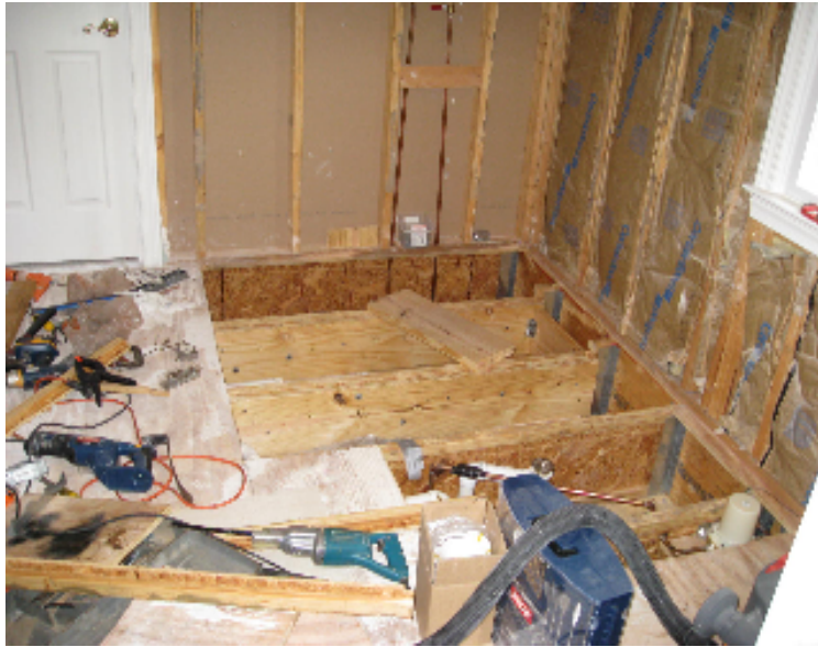
Picture 1: Gutted walls , floor to be recessed and after floor joists got reinforcement and a new plywood base
