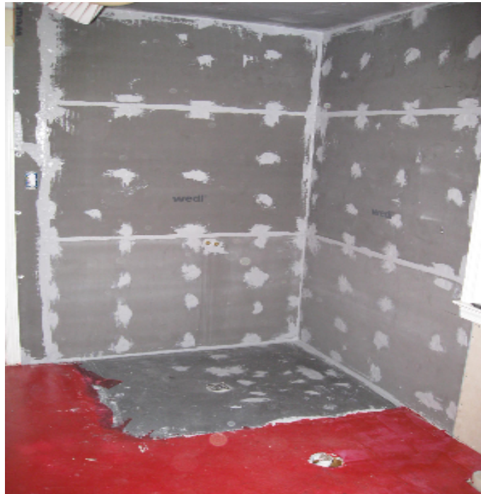
Picture 2: wediFundo base is and wedi walls are installed. No curb was used for this shower and waterproofing covers the floor surrounding the shower and is overlapping into the wedi base. Where floor height allows, the waterproof wedi building panel 1/4" or 1/2" can be used instead of a liquid membrane as shown in this picture. This way the surface can be leveled, provides insulating value and an excellent cementitious bond surface for tile and modified tile adhesive
